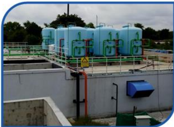
SEWAGE TREATMENT PLANT
